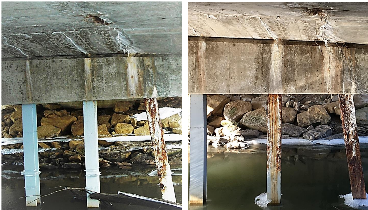
FIGURE 1: Corrosion of Highway 19 Yahara River Bridge. March of 2013 on left, December of 2019 on right. Stalactites form at the largest fracture every winter and slowly dissolve over the remainder of the year.
